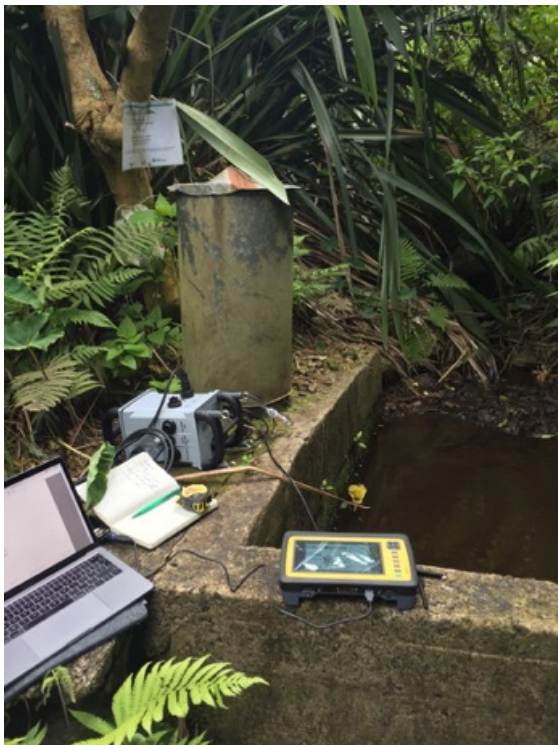
Plate 3.3: Blue Siren Flow Logger Installation at Grapevine Gut
