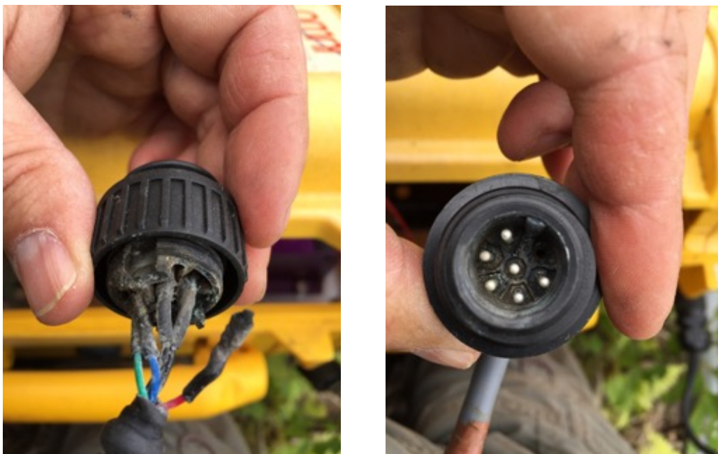
Plate 3.1: Corroded Weather Station Data Cables
